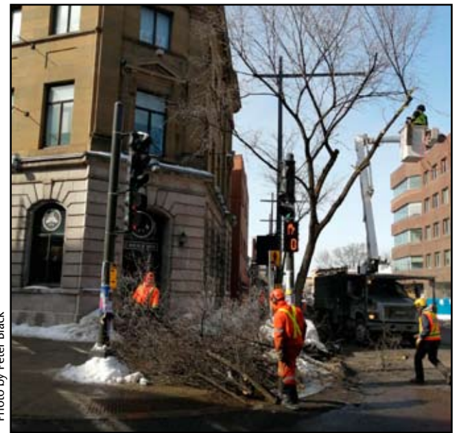
Workers take down a tree at the corner of Rue Dorchester and Rue Saint-Joseph to clear the way for construction of the tramway line.
